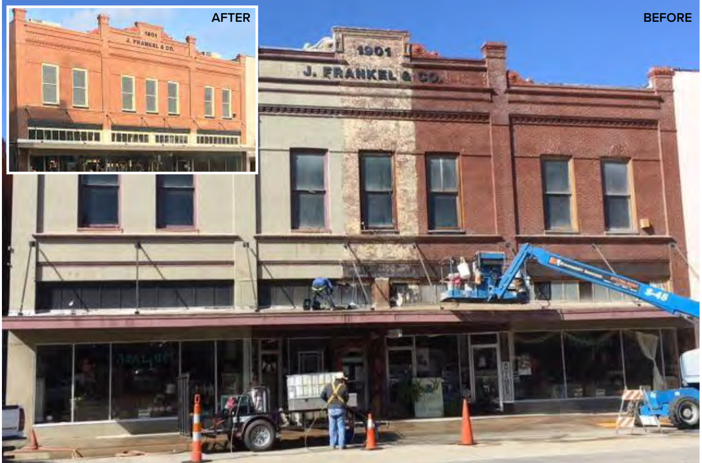
MAIN STREET FACADE GRANT Before and After images of facade restoration of a historic building at Crowley, LA
